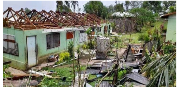
Cyclone Lola Damage
